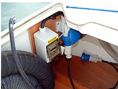
Shore power socket
