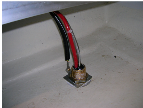
Exchanger - Under saloon floor To port
