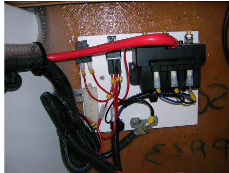
Operation relay Under the bed - Forward cabin
