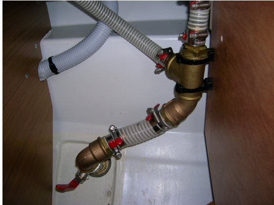
Drainage - Galley sink + Draining rack - behind the rubbish holder
