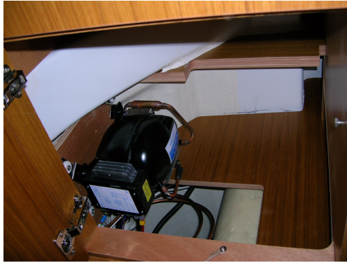
Refrigeration unit - Under the kitchen cupboard
