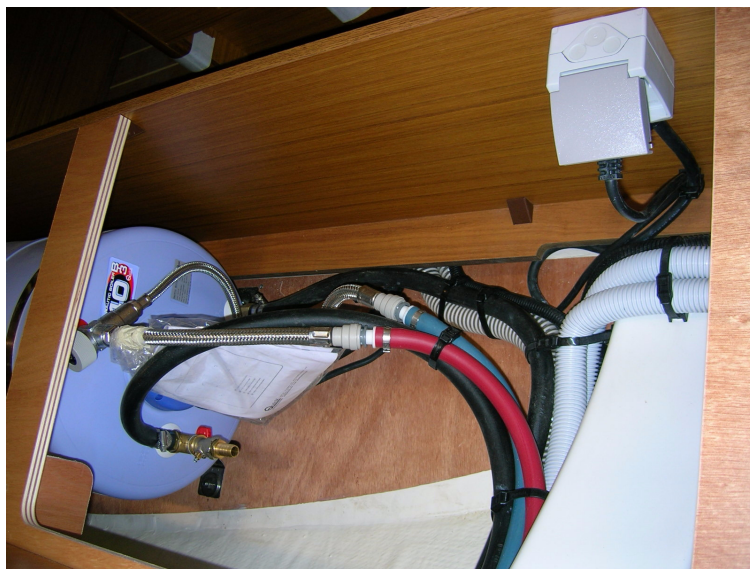
Socket 220V Water heater - Under saloon seating starboard
