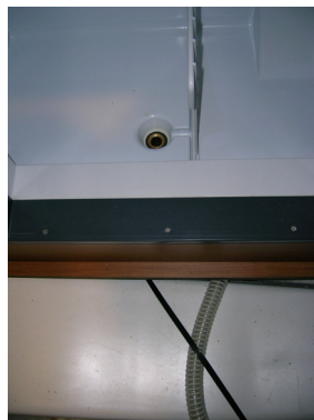
Drainage Fridge - In the sump well
