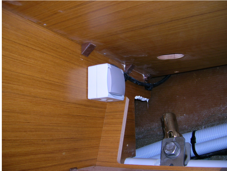
220V socket for micro wave oven - Under the kitchen cupboard
