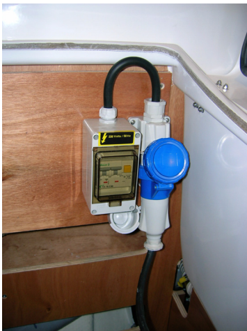
Breaker - Port aft locker
