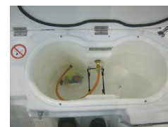
Gas cylinder locker (Reference 2)
