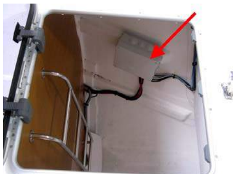
Operation relay Location: Sail locker
