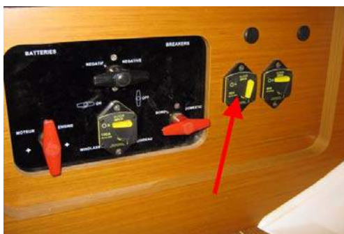
Breaker (30A) Location - Port aft cabin (Ref 1)
