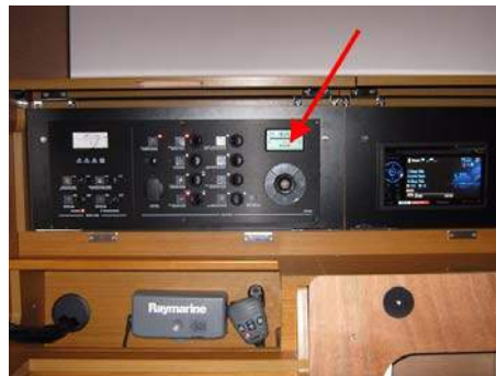
Gauge (on the electrical panel)
