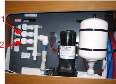
Water tank direction valves
