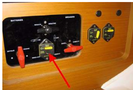
Breaker - 100A Location: Port aft cabin
