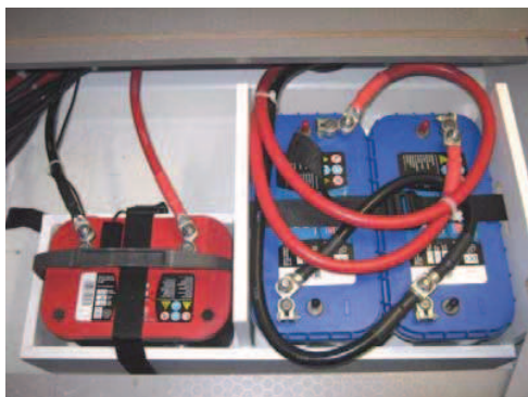
Generator battery - 50A Engine batteries - 2 x 75A
