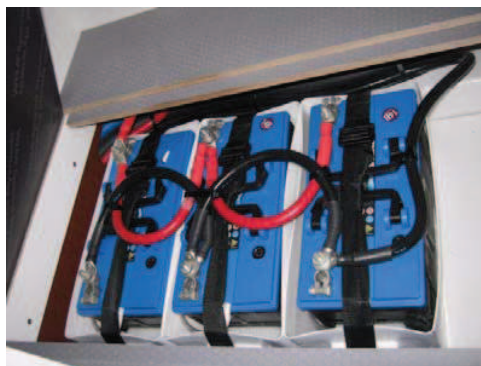
Service battery - 3 x 115A Spare service battery - 115A
