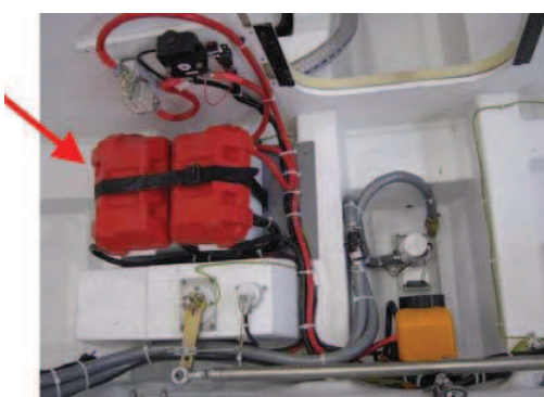
Batteries - Stern thruster - 2 x 50A
