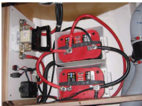
Bow thruster batteries - 2 x 50A
