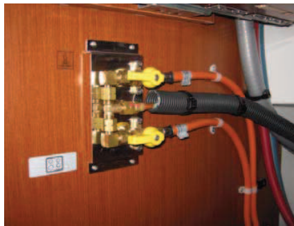
Gas supply valve
