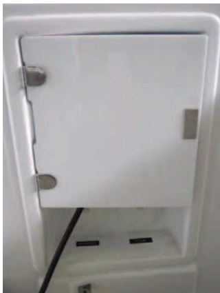
AC shore socket & Air conditioning (Ref 1)
