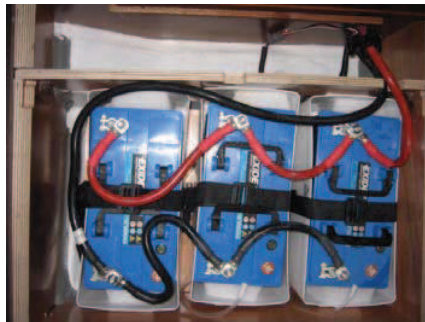
Service batteries: 2 x 115A Spare service batteries: 1 x 115A
