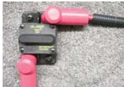
Figure 4-7. Main Circuit Breaker
