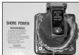
TYPICAL SHORE POWER INLET
