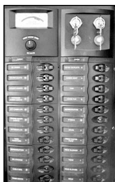
12-VOLT DC MAIN DISTRIBUTION PANEL
