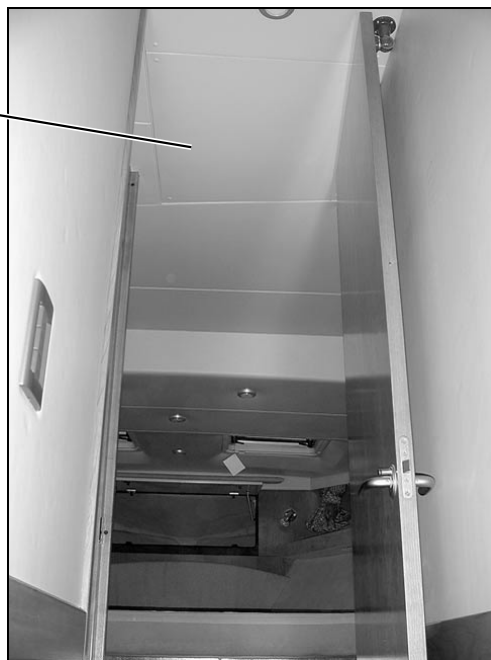
CEILING ACCESS PANEL
