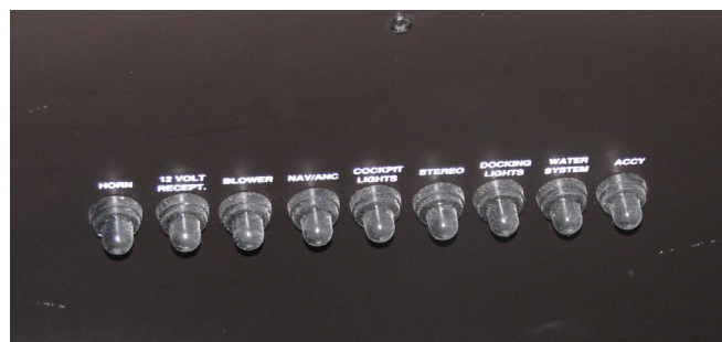
224FSC Helm Circuit Breaker Panel
