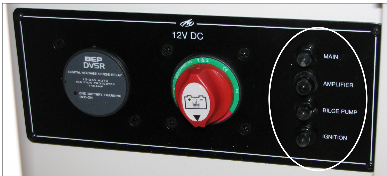
264FSC Battery Switch Circuit Breaker Panel
