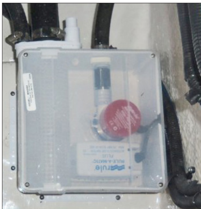
Sump Pump System
