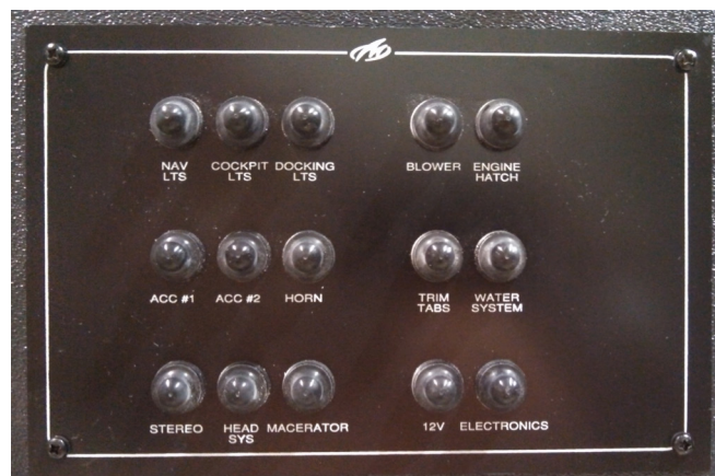
264 FSC Helm Circuit Breaker Panel
