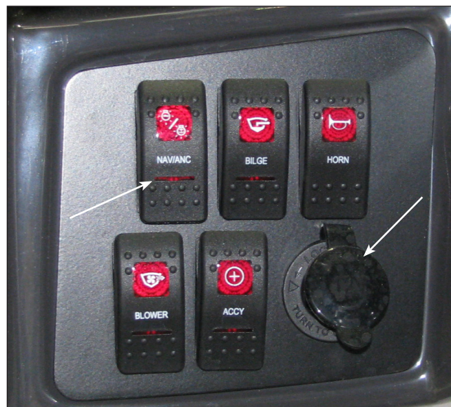
Helm Switches Showing LED Lights & 12 Volt Accessory Plug
