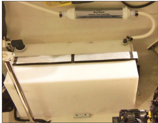
Typical Holding Tank & Charcoal Filter in Bilge
