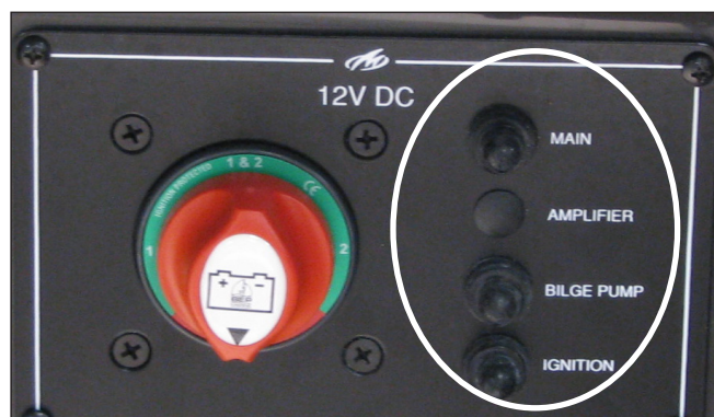
196MS Battery Switch Circuit Breaker Panel
