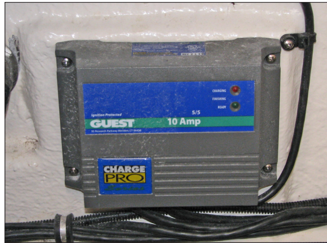
Typical Battery Charger
