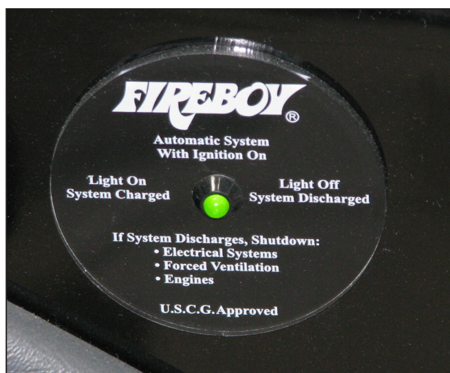
Fire Extinguisher Panel In Helm
