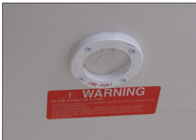
Typical Fire Port
