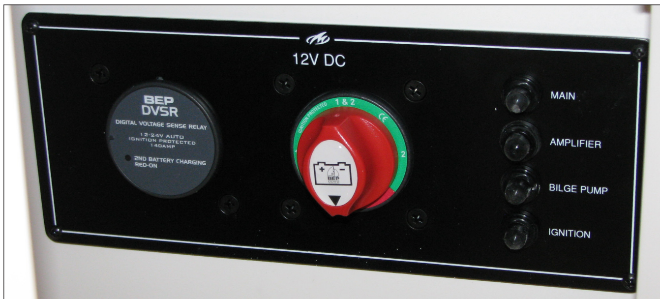
Typical Dual Battery Selector Switch Panel with DVSR
