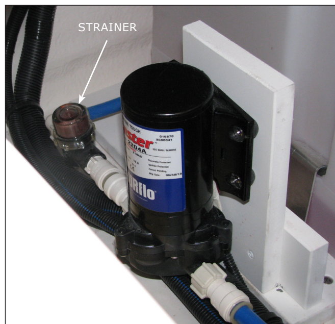
Typical Water Pump & Strainer
