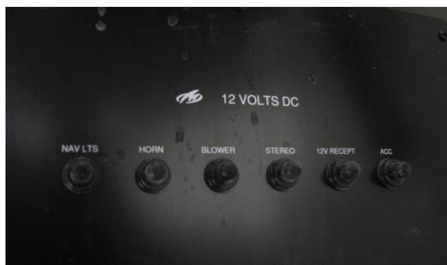
196 MFS Helm Circuit Breaker Panel
