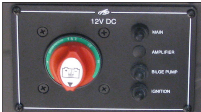
Typical Dual Battery Selector Switch Panel No Digital Voltage Sensitive Relay
