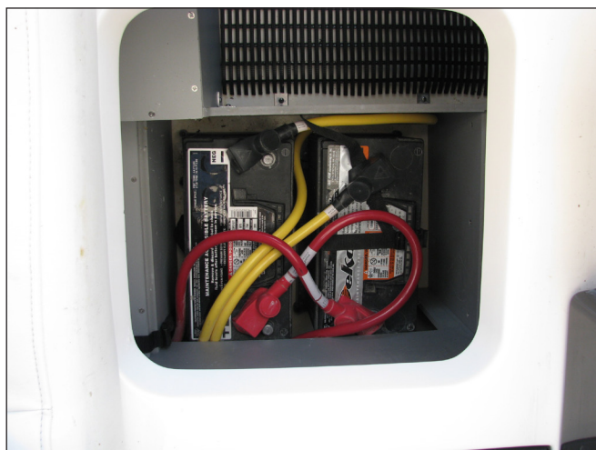
288SS Batteries In Aft Bench Seat Compartment
