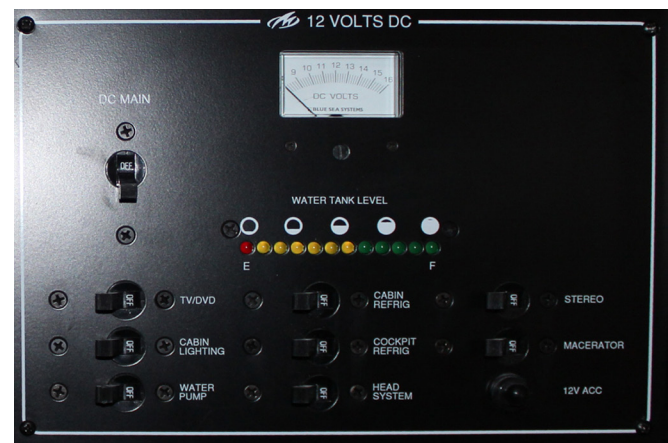
Cabin DC Electrical Panel
