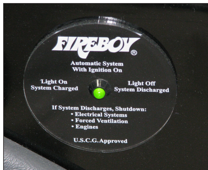
Fire Extinguisher Panel In Helm
