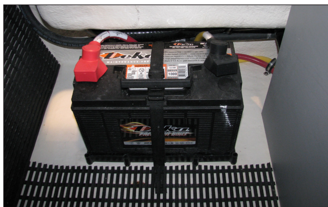
268SS Battery Installation
