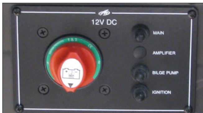
Typical 268SS Dual Battery Switch Panel
