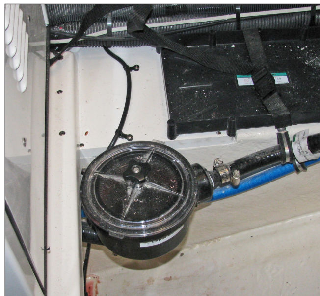
Air Conditioner Pump & Strainer
