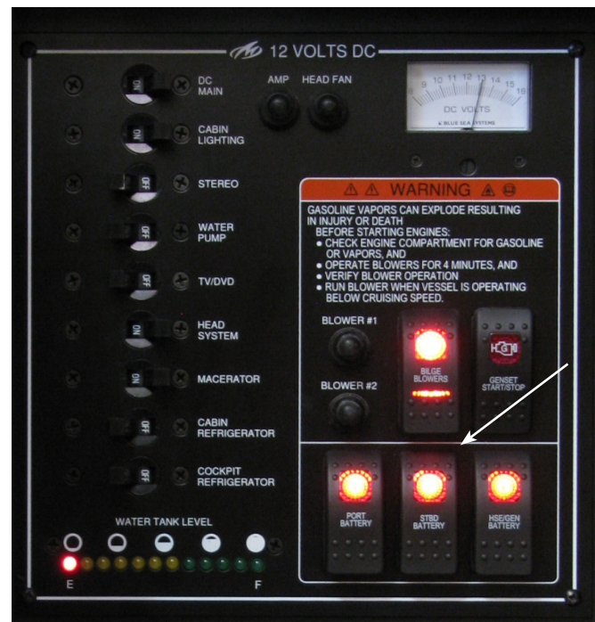
Remote Battery Switches in Cabin DC Panel
