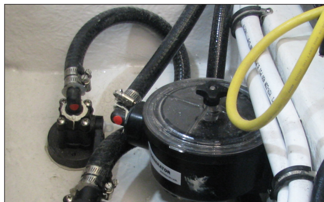
Generator Sea Strainer & Seacock
