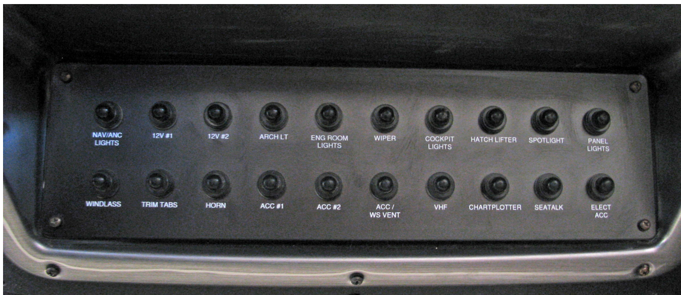
315SY Helm Circuit Breaker Panel
