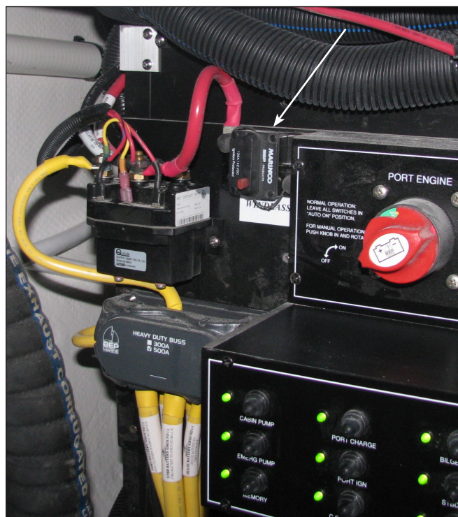
Windlass Main Circuit Breaker
