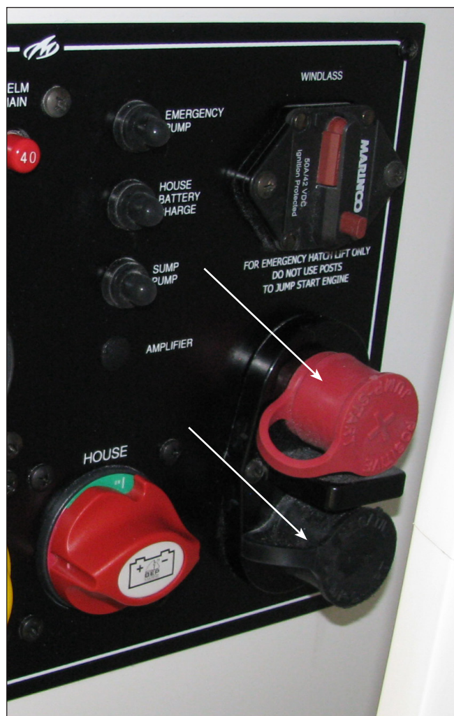
Battery Switch Jumper Terminals
