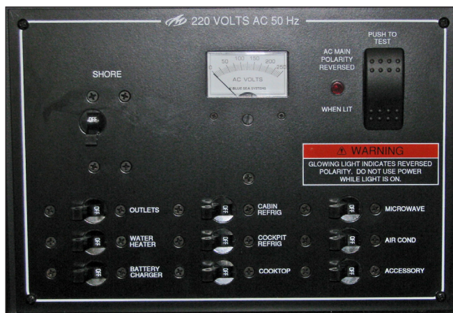
275/295SY AC Circuit Breaker Panel - 220 Volt/50 Hz
