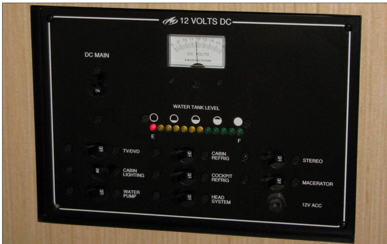
275/295SY Cabin DC Circuit Breaker Panel
