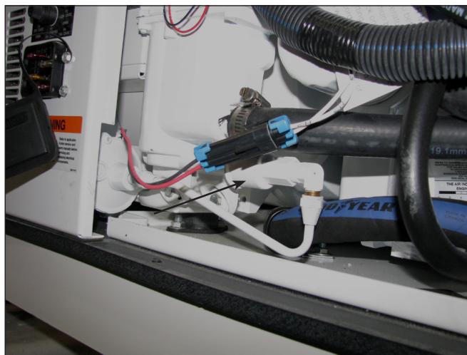
Typical Generator Fuel Filter
