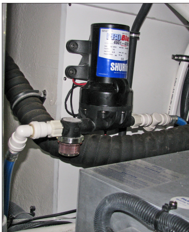
Fresh Water Pump & Strainer
