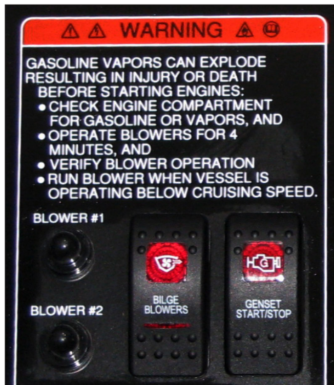
Generator Remote Control Panel in Cabin
