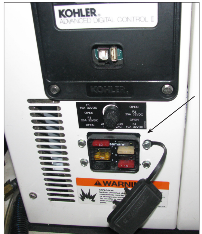
Typical Generator DC Circuit Fuse Panel
