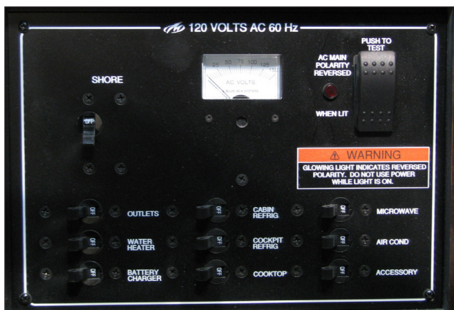
275/295SY AC Circuit Breaker Panel - 120 Volt/60 Hz
