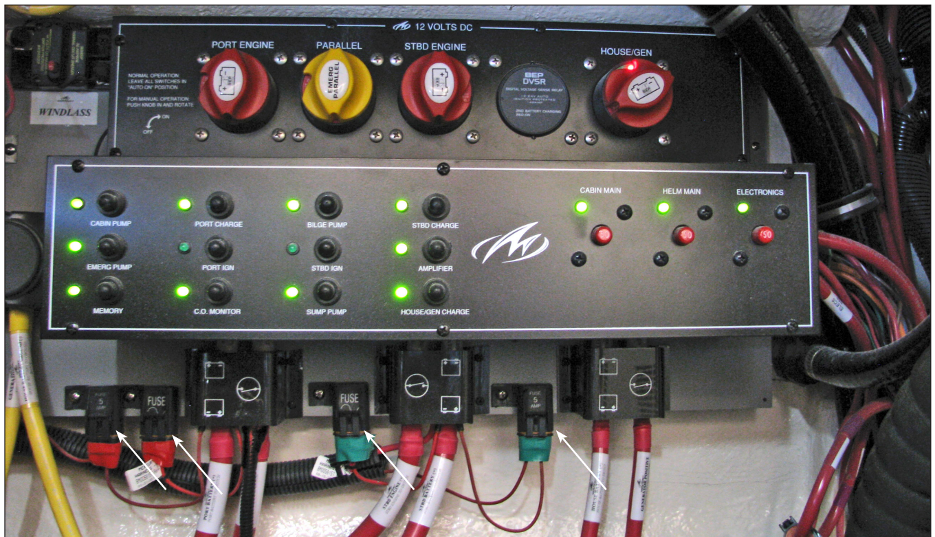
Typical 315SY Battery Switch Panel & Mercruiser Fuses
