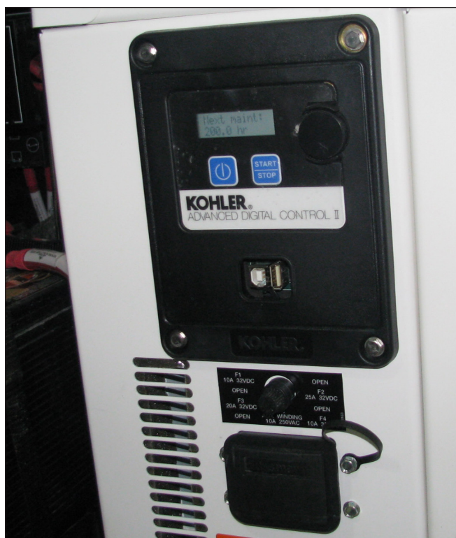
Typical Generator Control Panel
