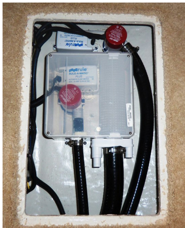
Forward Bilge Pump & Automatic Switch
