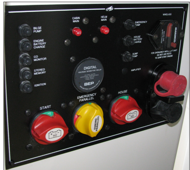
275/295SY Battery Switch Panel
