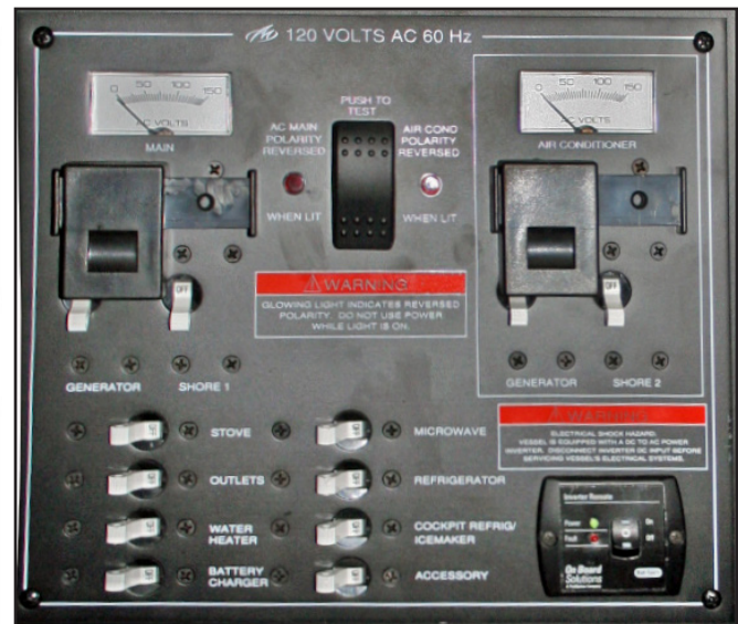
AC Accessory Breaker Panel
