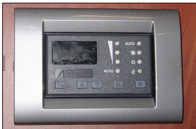
Air Conditioner Control Panel
