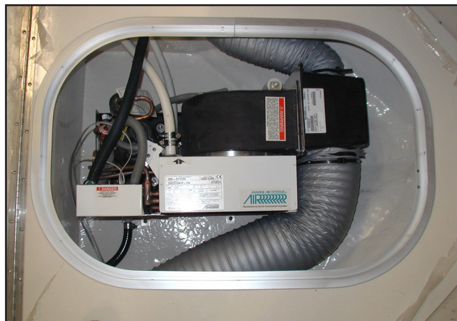
Air Conditioner Below V-Berth
