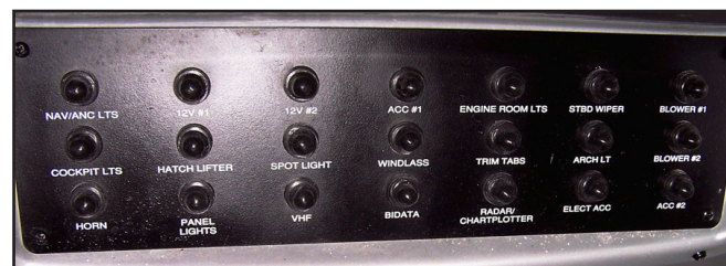
Helm Switch Breaker Panel
