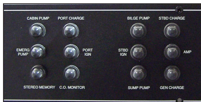
Battery Switch Breaker Panel
