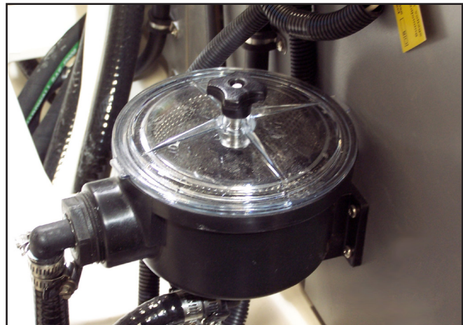
Generator Sea Strainer
