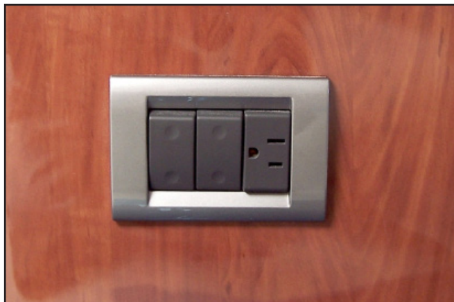
Typical Cabin Switch Panel and GFI Outlet
