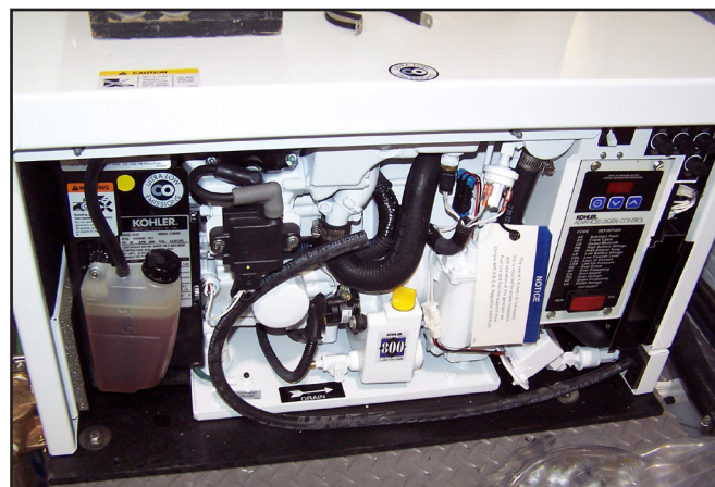
Typical Gasoline Generator
