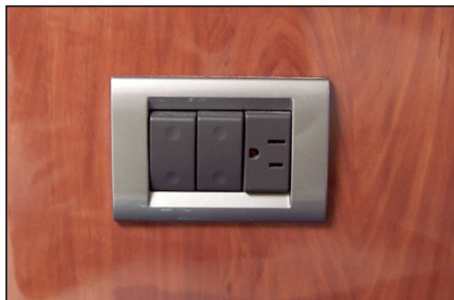
Typical Cabin Switch Panel and GFI Outlet
