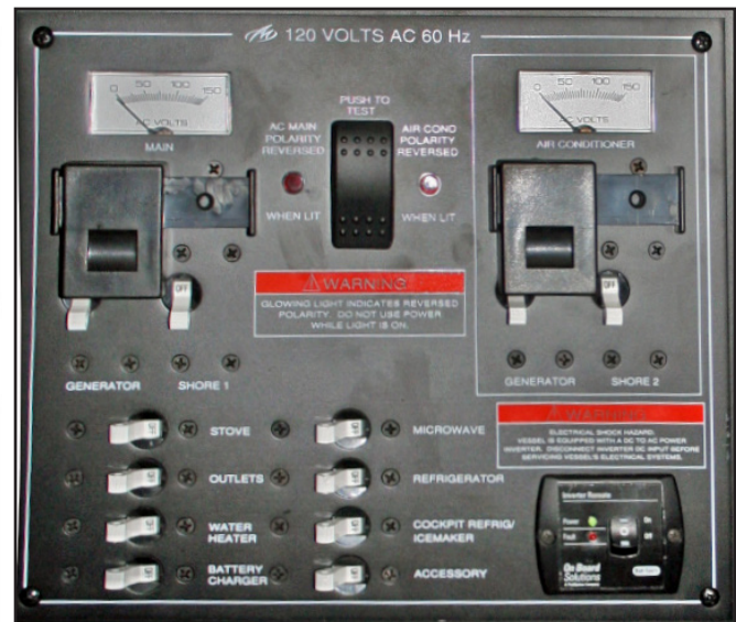
AC Accessory Breaker Panel
