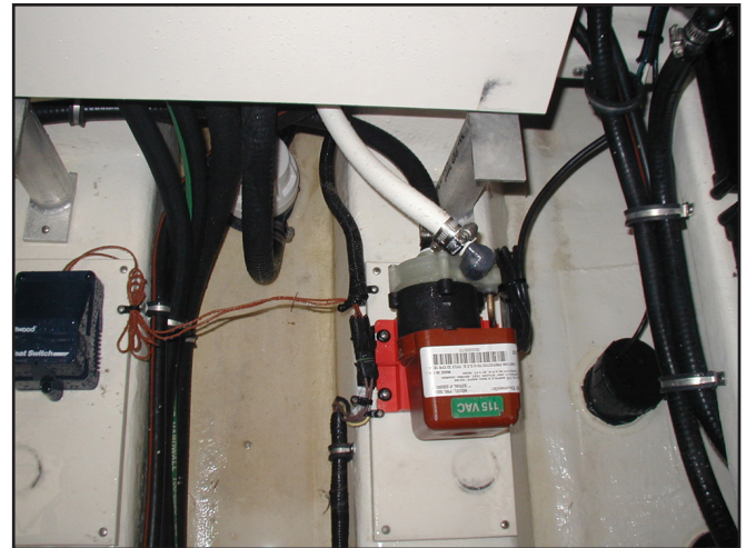
Air Conditioning Pump
