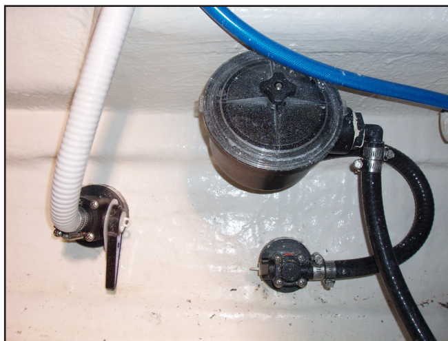
Holding Tank Overboard Discharge Thru-Hull Valve
