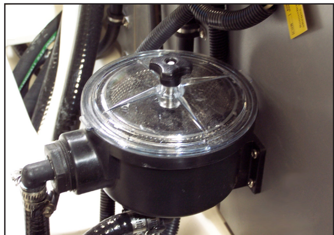
Generator Sea Strainer
