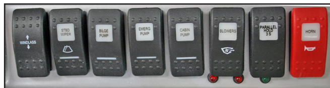
Helm Switch Panel - Starboard Side
