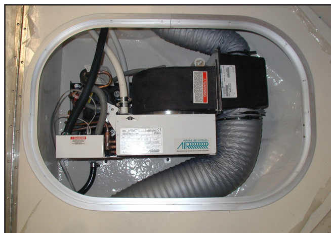
Air Conditioner Below V-Berth
