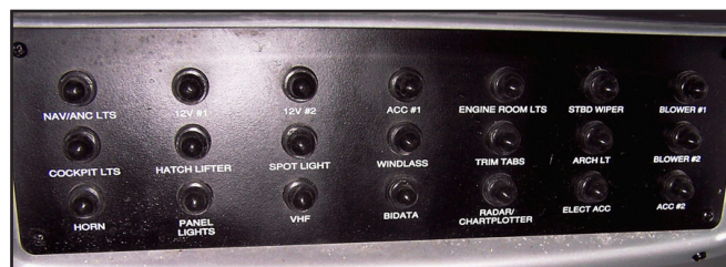
Helm Switch Breaker Panel
