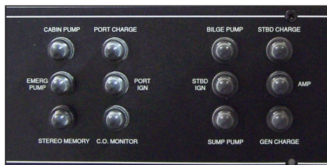
Battery Switch Breaker Panel
