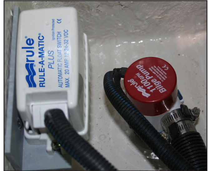
Typical Bilge Pump and Automatic Float Switch
