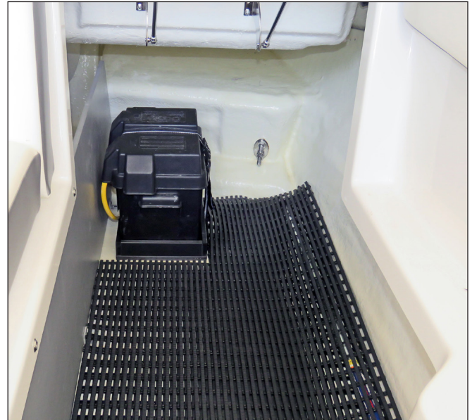
Battery Location In Storage Compartment
