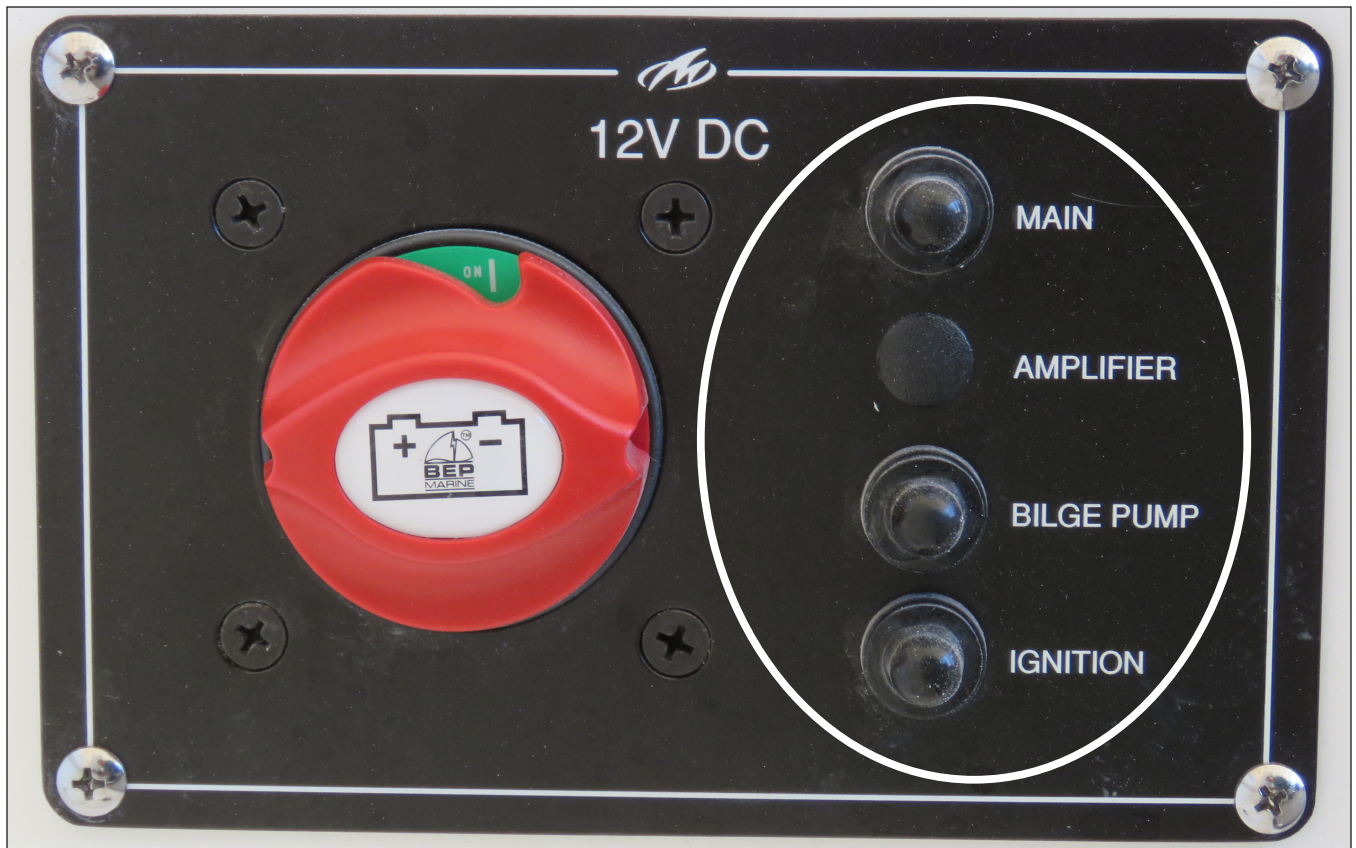
Battery Switch Panel Circuit Breakers
