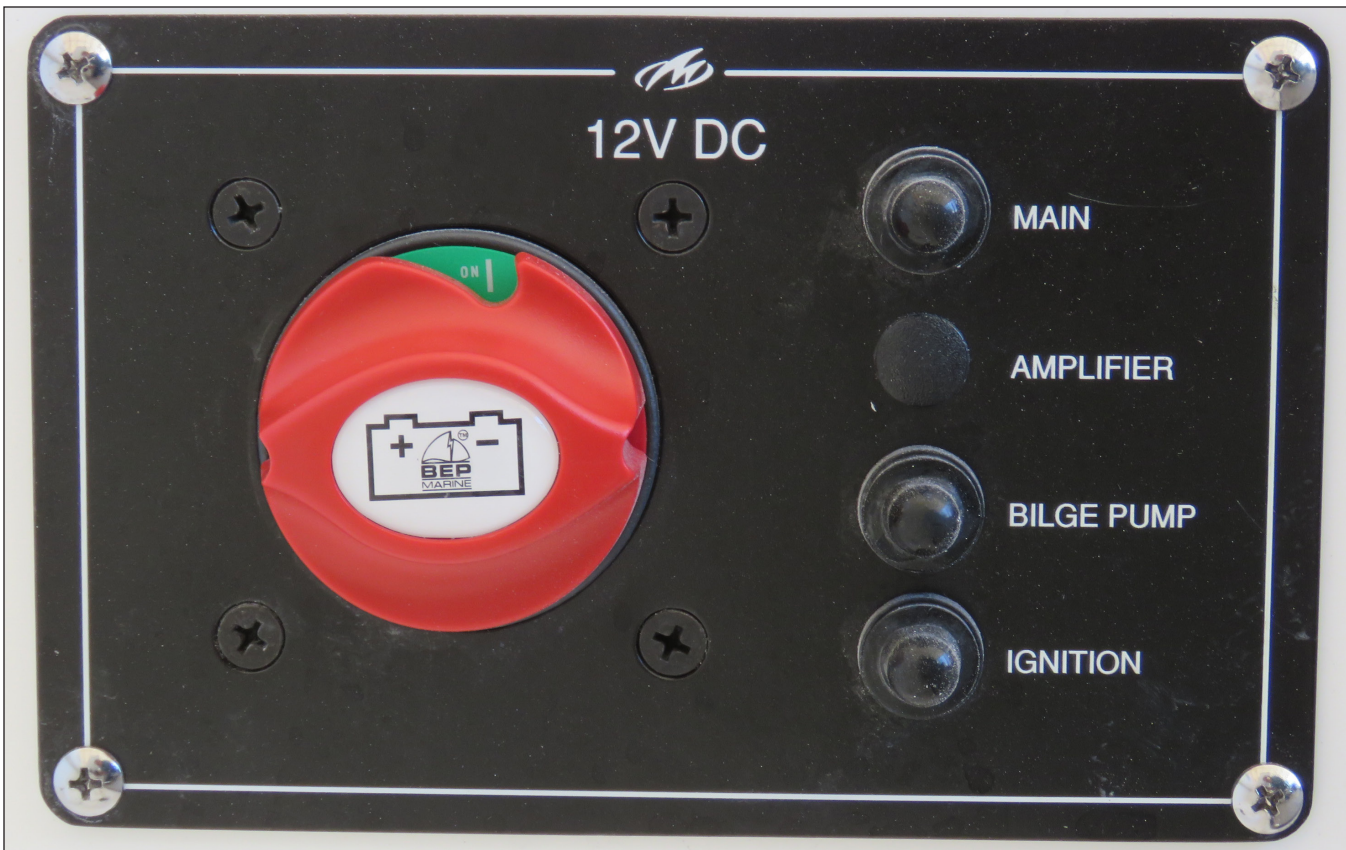
Battery Switch & Circuit Breakers
