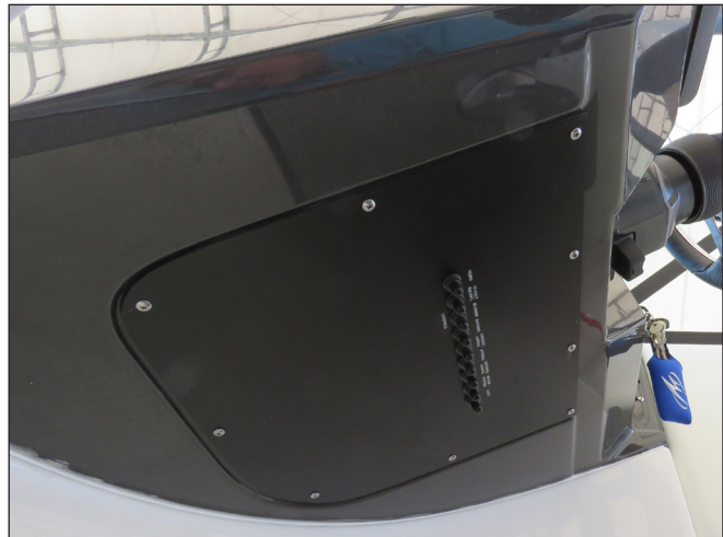
Removable Circuit Breaker Panel
