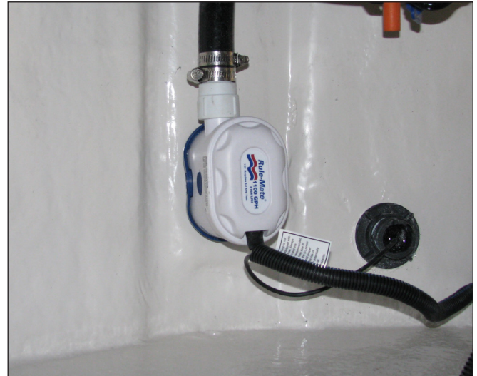
Typical Automatic Bilge Pump
