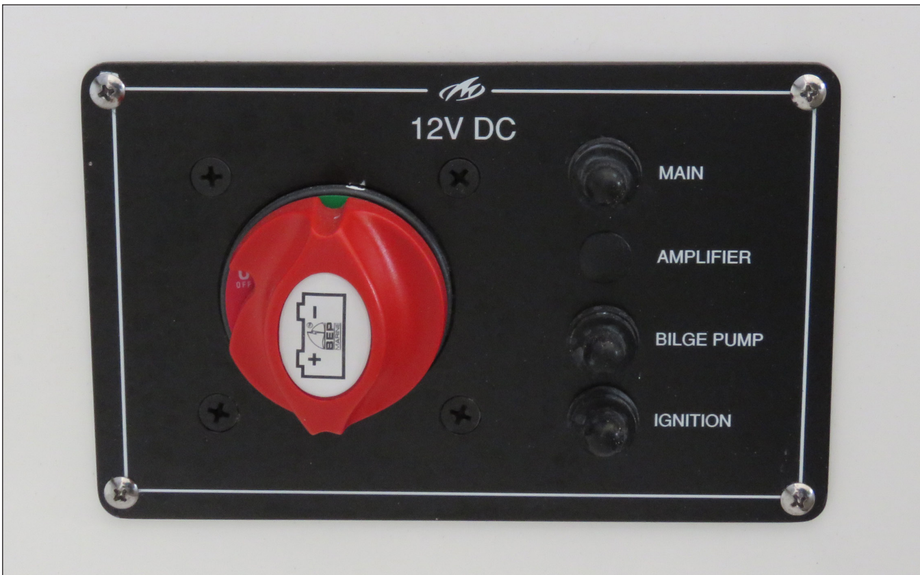
Battery Switch & Circuit Breakers
