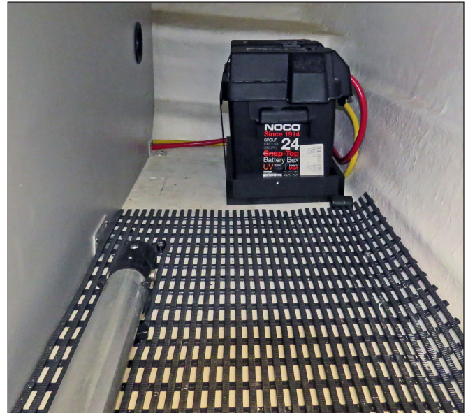
Battery Location In Storage Compartment
