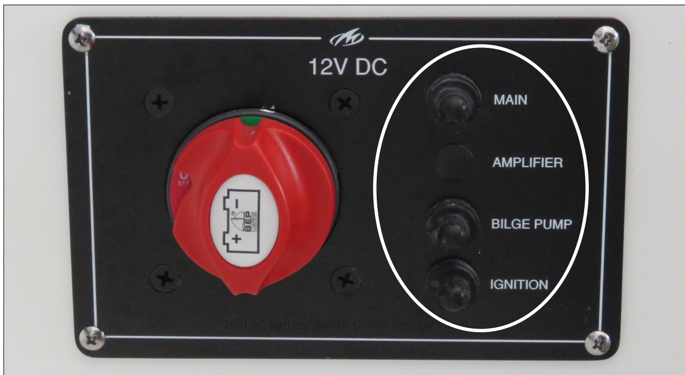
Battery Switch Panel & Circuit Breakers
