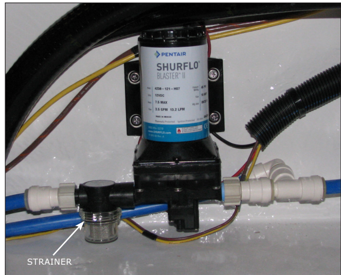
Fresh Water Pump & Strainer
