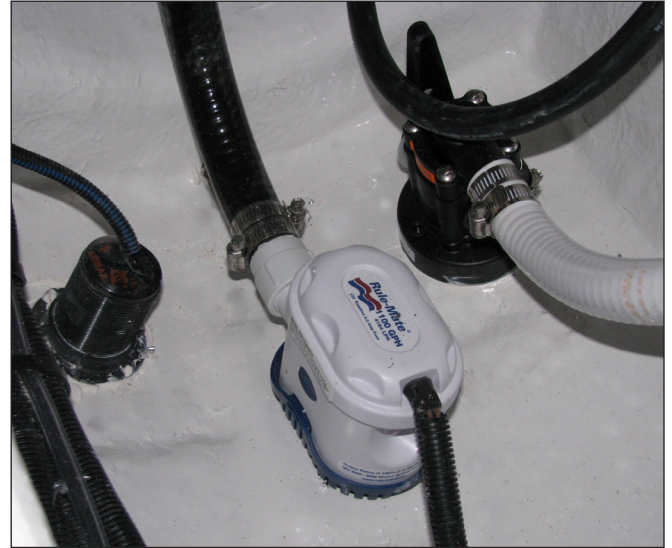
Typical Bilge Pump with Automatic Float Switch
