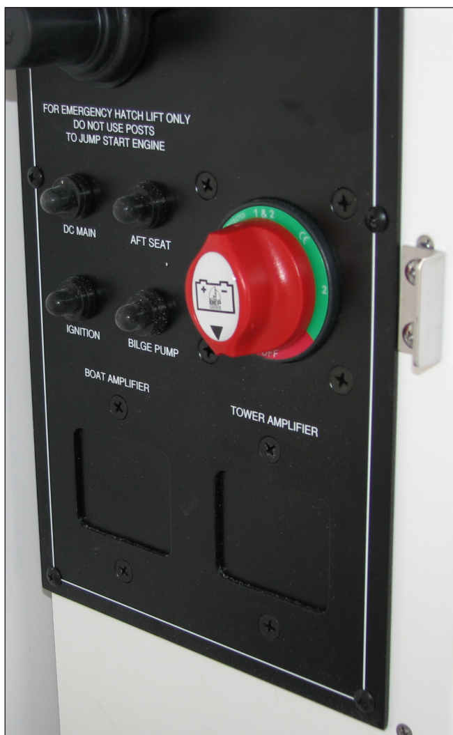
Battery Switch Panel Circuit Breakers
