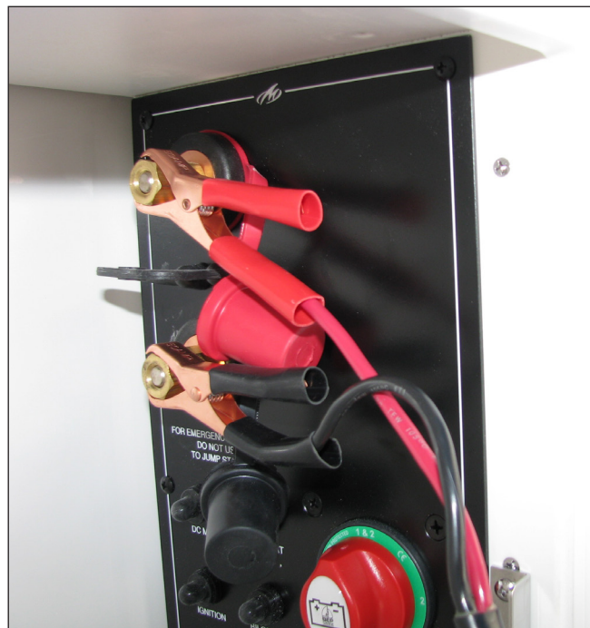
Jumper Harness Connected To Terminals
