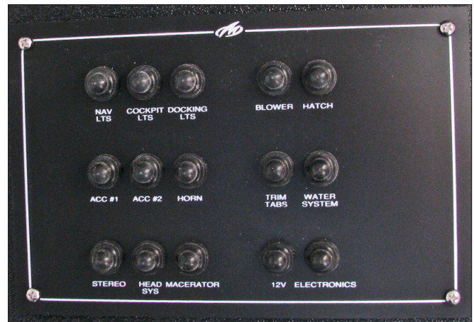
Main Helm Switch Circuit Breaker Panel
