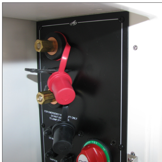
Access Hatch Jumper Terminal - Caps Removed
