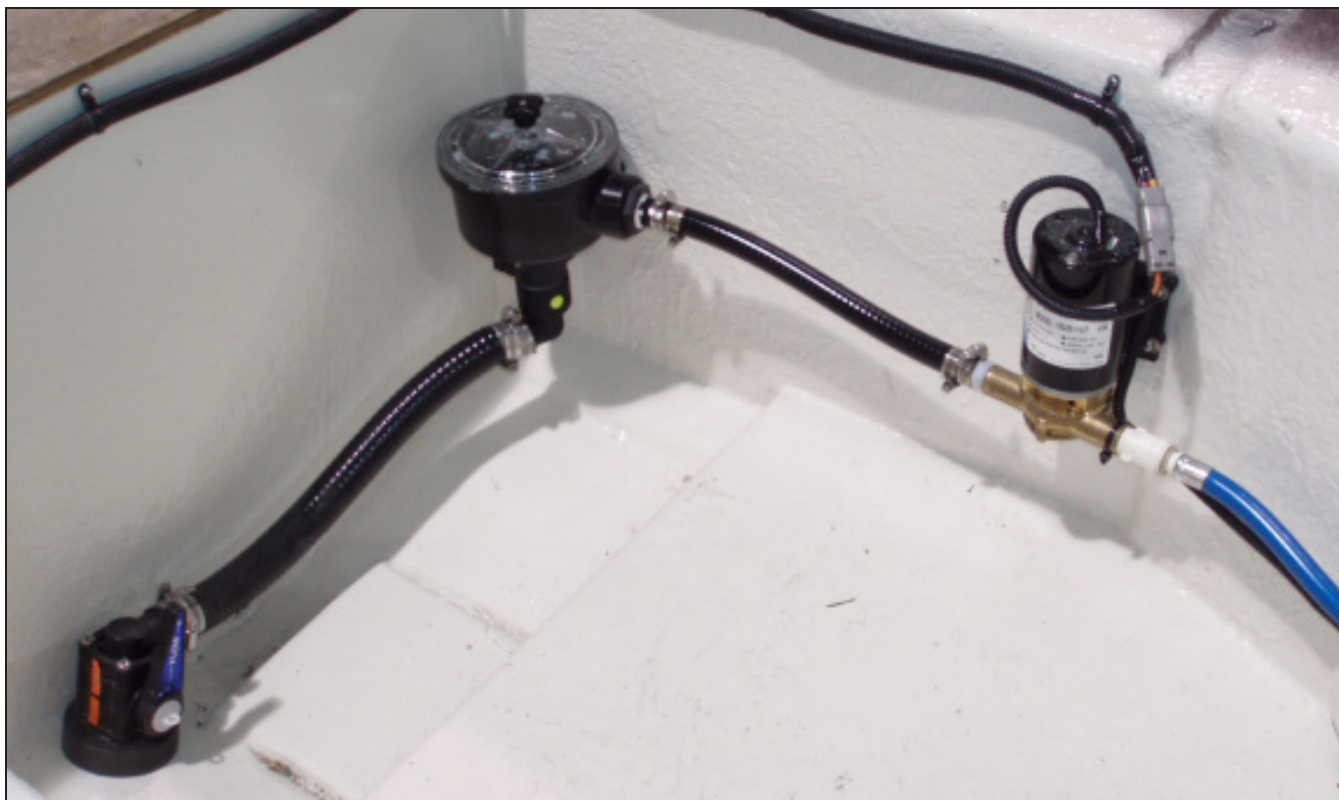
Ballast Pump Water System
