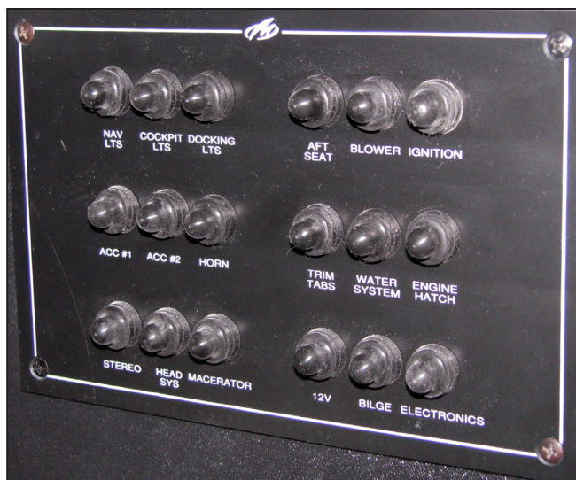
Typical Main DC Circuit Breaker Panel
