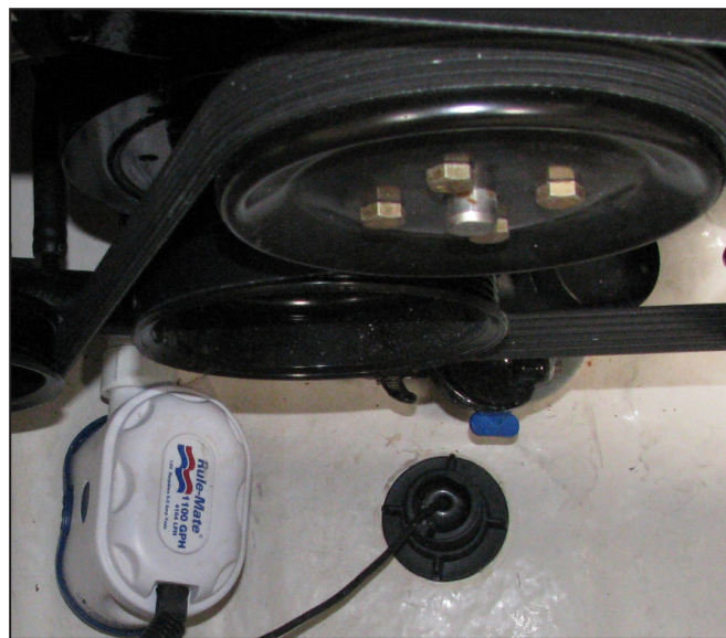
Typical Bilge Pump with Automatic Float Switch
