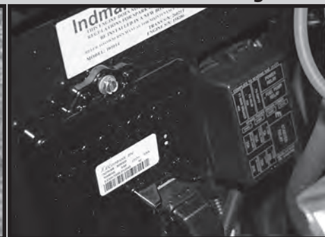
Fuse Panel - Back of Engine
