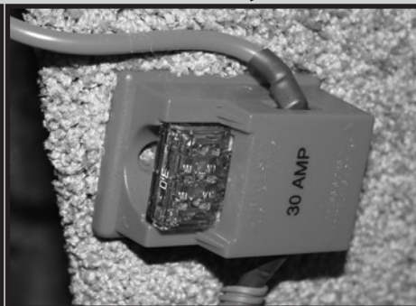
Fuse Panel - Battery Connection
