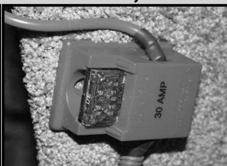
Fuse Panel - Battery Connection
