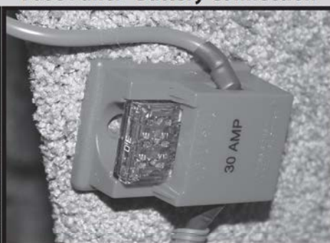
Fuse Panel - Battery Connection
