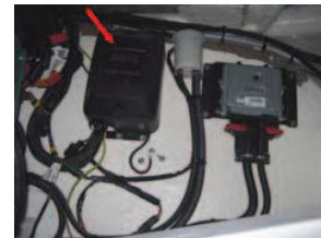
Electronics box - Joystick Location: Engine compartment
