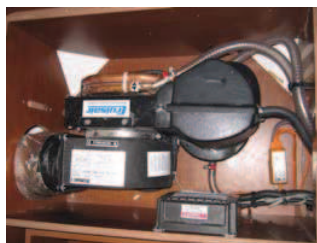
Compressor - Forward cabin (Reference 7)
