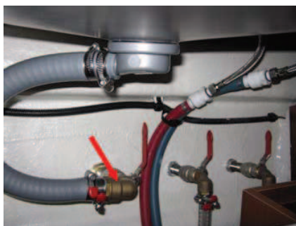
Galley draining - Sink
