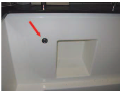
Drainage pump control - Shower
