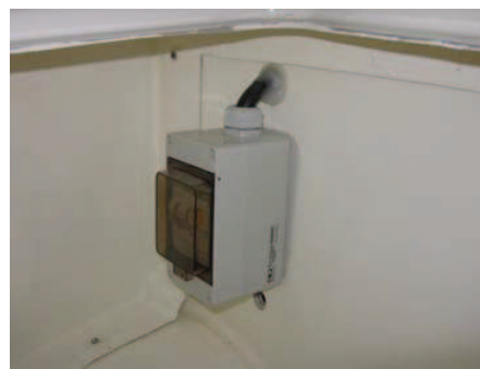
Breaker 220V 32A (Reference 2)
