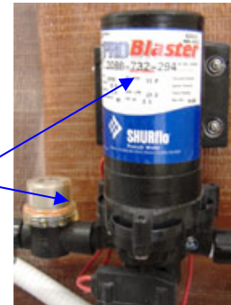
Fresh Water Pump and Filter
