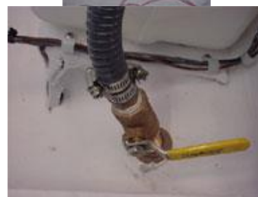
Seacock is shown in the closed position.
