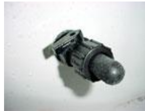
Lever on the aerator fitting is closed
