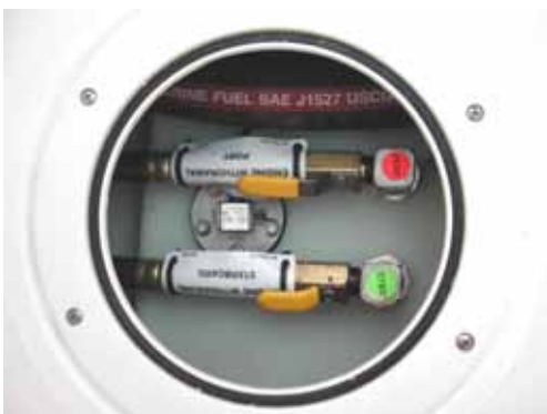
Fuel Valves Forward Tank (Typical)
