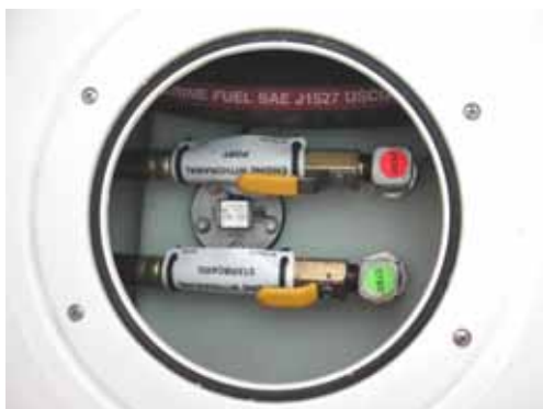
Fuel Valves Forward Tank (Typical)
