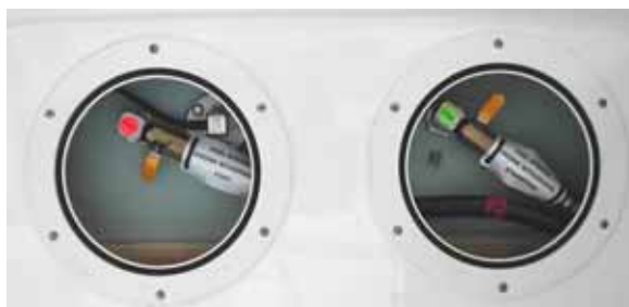
Fuel Valves Aft Tank (Typical)
