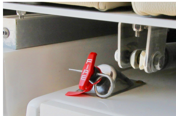
Fire system manual discharge
