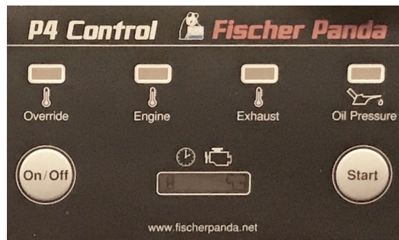
Generator control panel on the AC MDP
