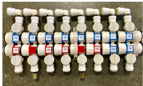
Water system manifold
