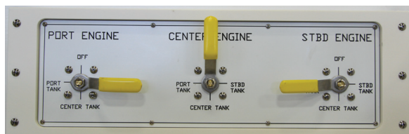
Fuel Manifold System
