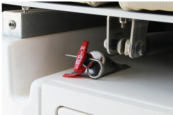
Fire System Manual Discharge
