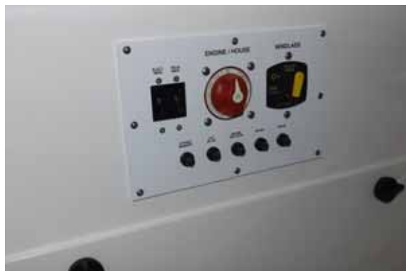
Battery Switches and Main Breakers
