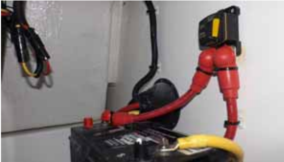
Main Battery Disconnect
