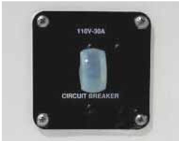
Shore Power Breaker
