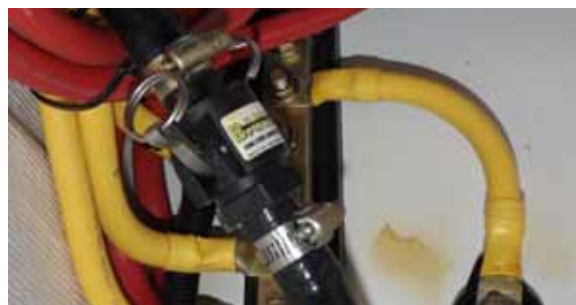
Rear Storage Drain
