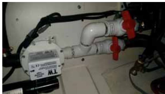
Fishbox Drain Valves
