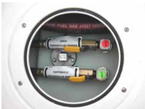
Fuel Valves Forward Tank (Typical)
