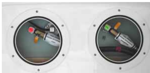
Fuel Valves Aft Tank (Typical)
