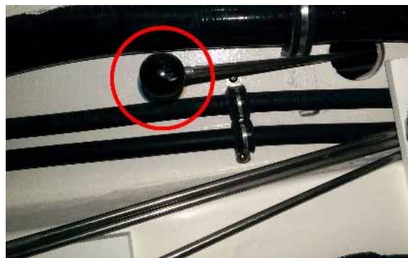
Deck drain ball valve levers
