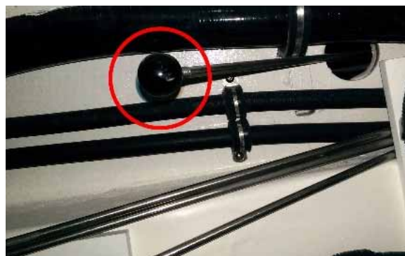
Deck drain ball valve levers
