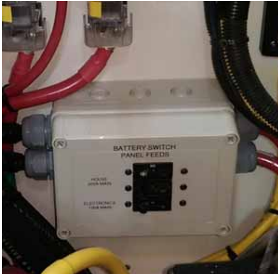
Main Electronics Battery Disconnect
