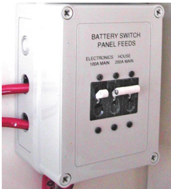
Battery Switch Panel Feeds
