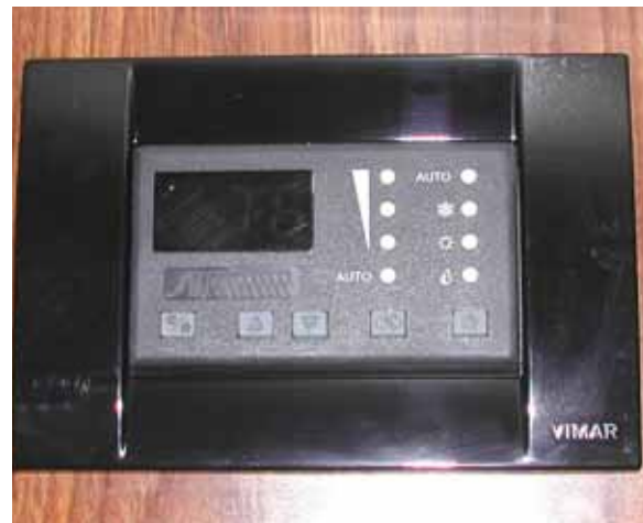
Air Conditioning Control Panel
