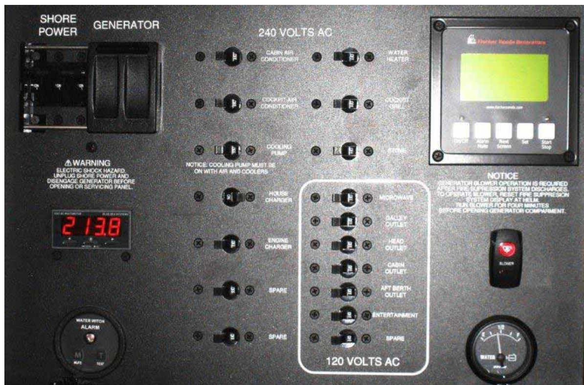
AC Main Distribution Panel (AC MDP)
