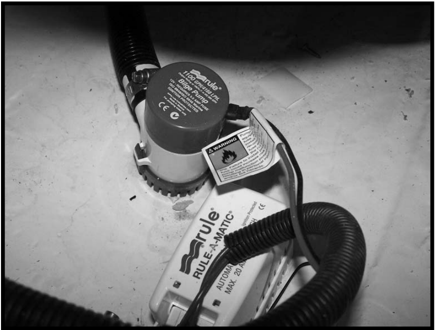
Typical Bilge Pump And Automatic Float Switch
