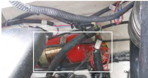
Typical Automatic Fire Extinguisher Canister Location
