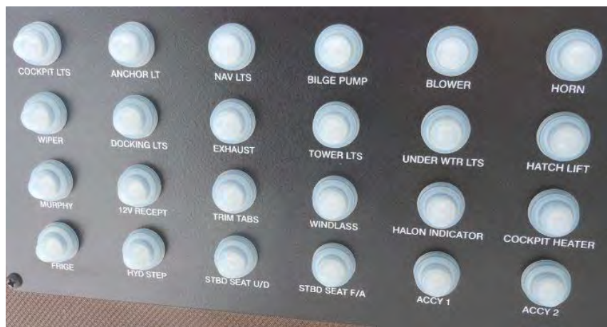
UNDER HELM BREAKER PANEL
