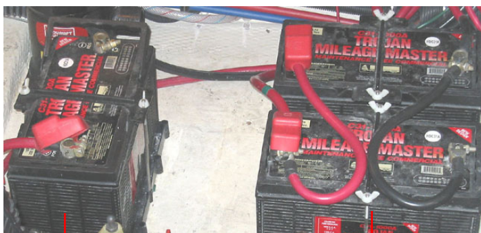
PORT ENGINE CRANKING BATTERY
