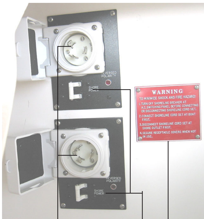
TYPICAL SHORE POWER INLETS
