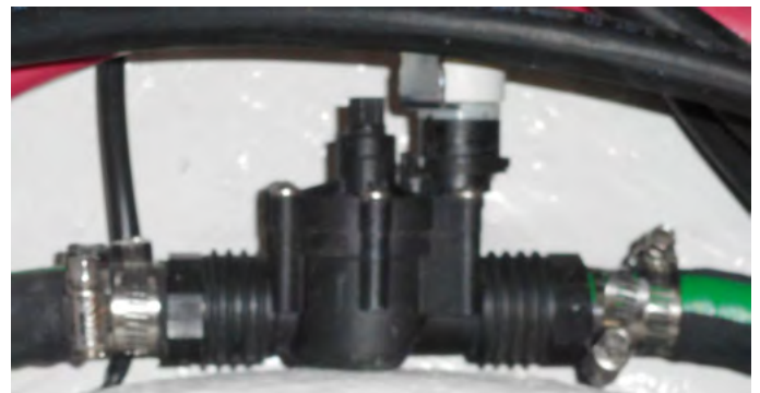
GENERATOR IN-LINE VALVE
