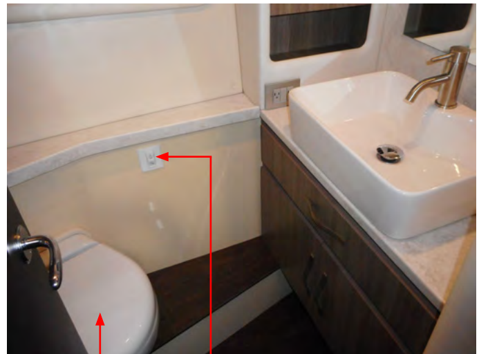
VACUUM STYLE TOILET
