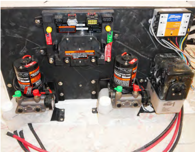
TYPICAL POWER STEERING BOARD
