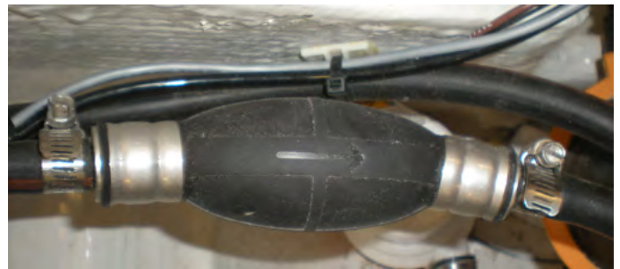
FUEL PRIMER BULB IN SUMP AREA
