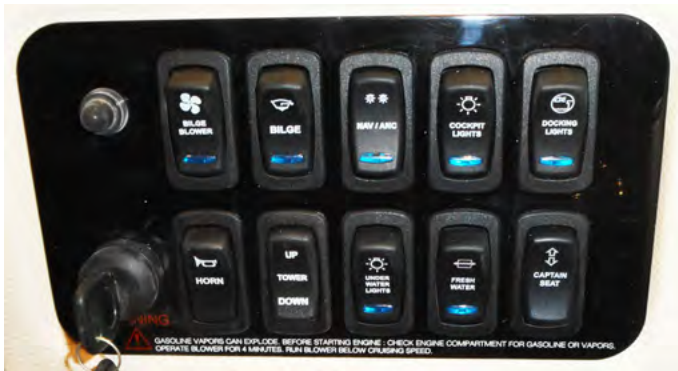
Typical Switch Panel Shown
