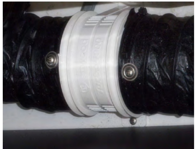
Typical Ventilation Blower with Hose
