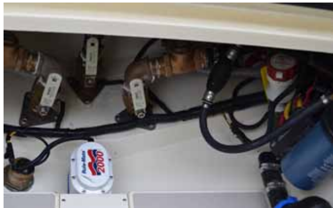
Bilge Pump and Baitwell Pumps
