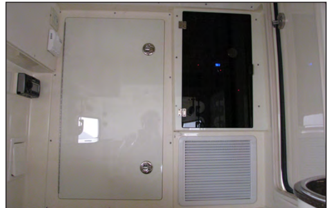
Cabin Breaker Panel and Helm Access Door
