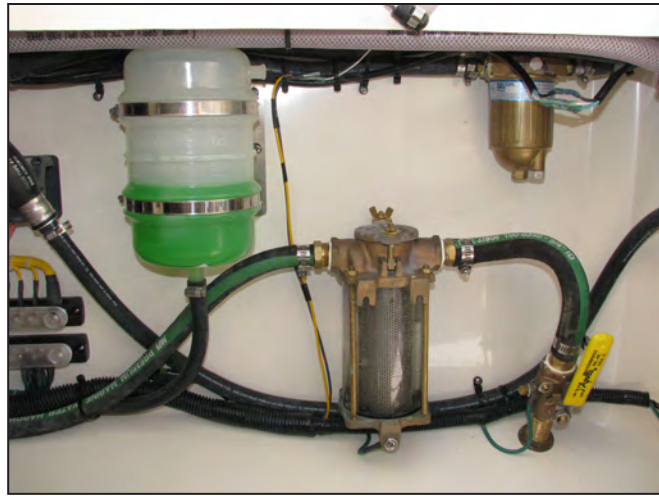
Generator Sea Strainer and Thru-Hull Valve
