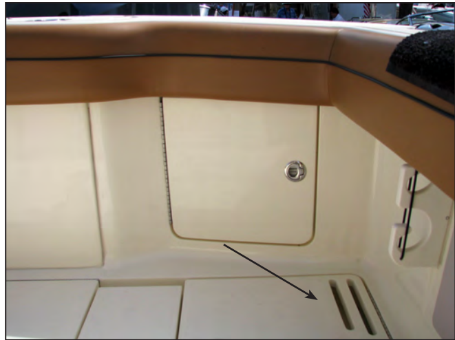
Port Side Cockpit Scupper
