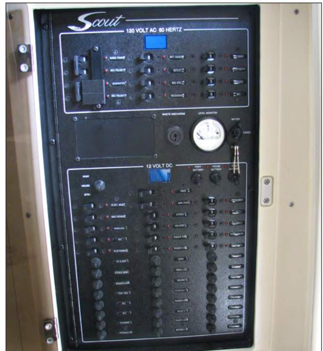
Cabin AC/DC Circuit Breaker Panel
