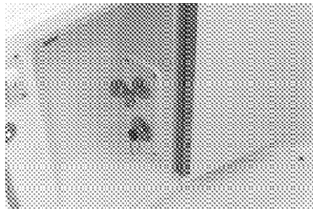
Fresh Water Washdown & Dockside Water Inlet (fig. 5.3.3)
