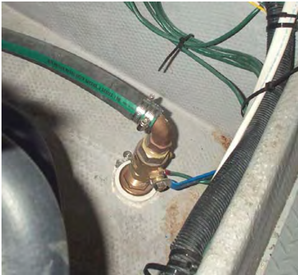
The photo above shows the valve closed.
