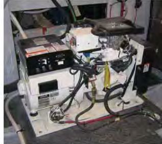
Generator: Located under the cockpit.
