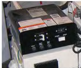
Breaker: Located on top of the Generator.
