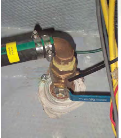
The photo above shows the valve closed.
