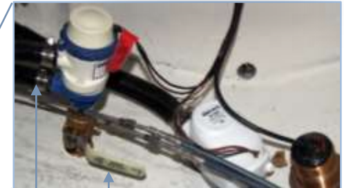
Shut Off Valve
