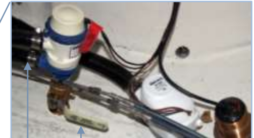
Shut Off Valve
